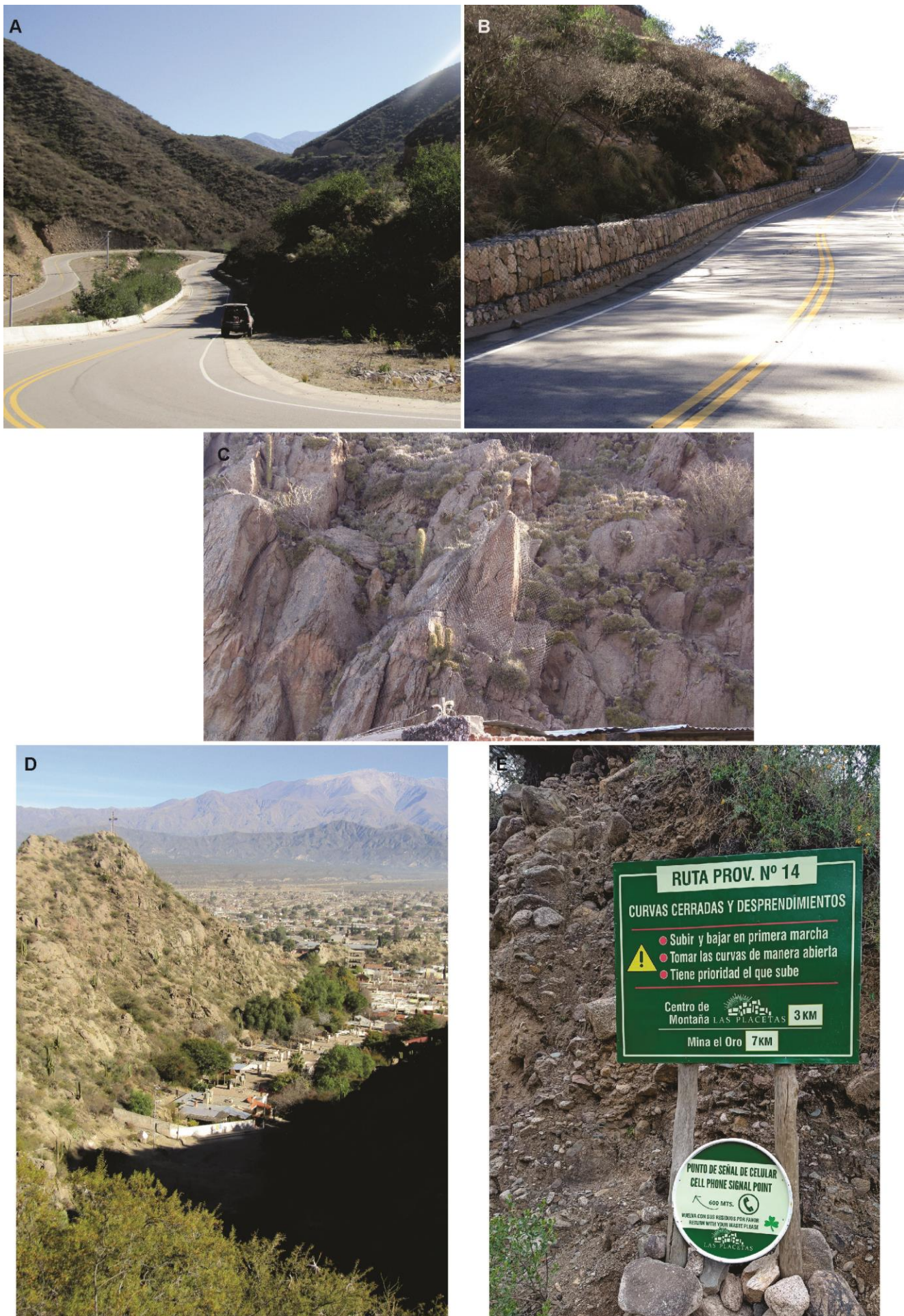
Fig. S13. Slope protection and retention structures. A–B) Retaining structures along Provincial Route 15 ( 29^{\circ}10'58''\text{S} / 67^{\circ}37'04''\text{W} ). C) Wire mesh installed near the roof of a building along Provincial Route 12 ( 29^{\circ}09'43''\text{S} / 67^{\circ}29'04''\text{W} ). D) Retention structure in the "El Rincón" neighborhood ( 29^{\circ}10'19''\text{S} / 67^{\circ}29'05''\text{W} ). E) Warning signage indicating a collapse-prone area ( 29^{\circ}05'53''\text{S} / 67^{\circ}41'51''\text{W} ).
