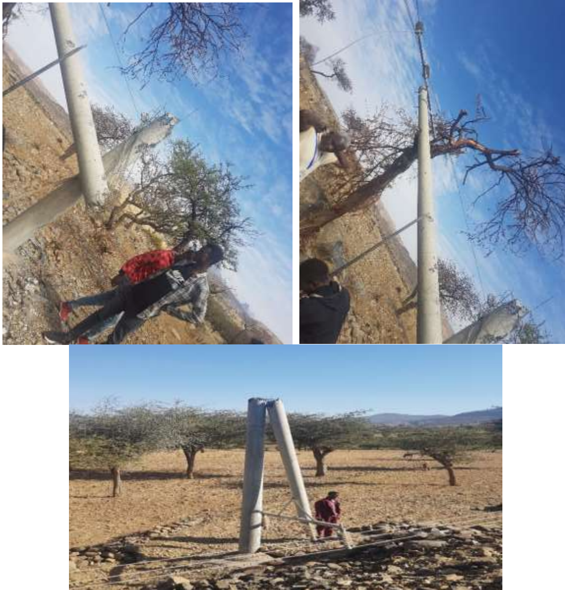
Fig.4.1: Cement pole line support failure during the war in Tigray [38]
