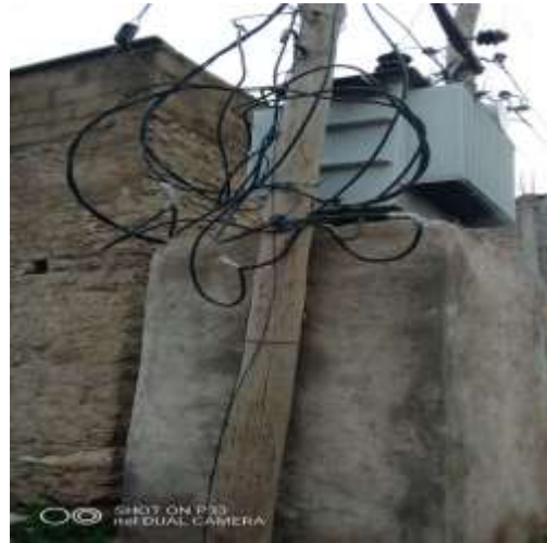
b) Distribution transformer without drop out Fuse Box
