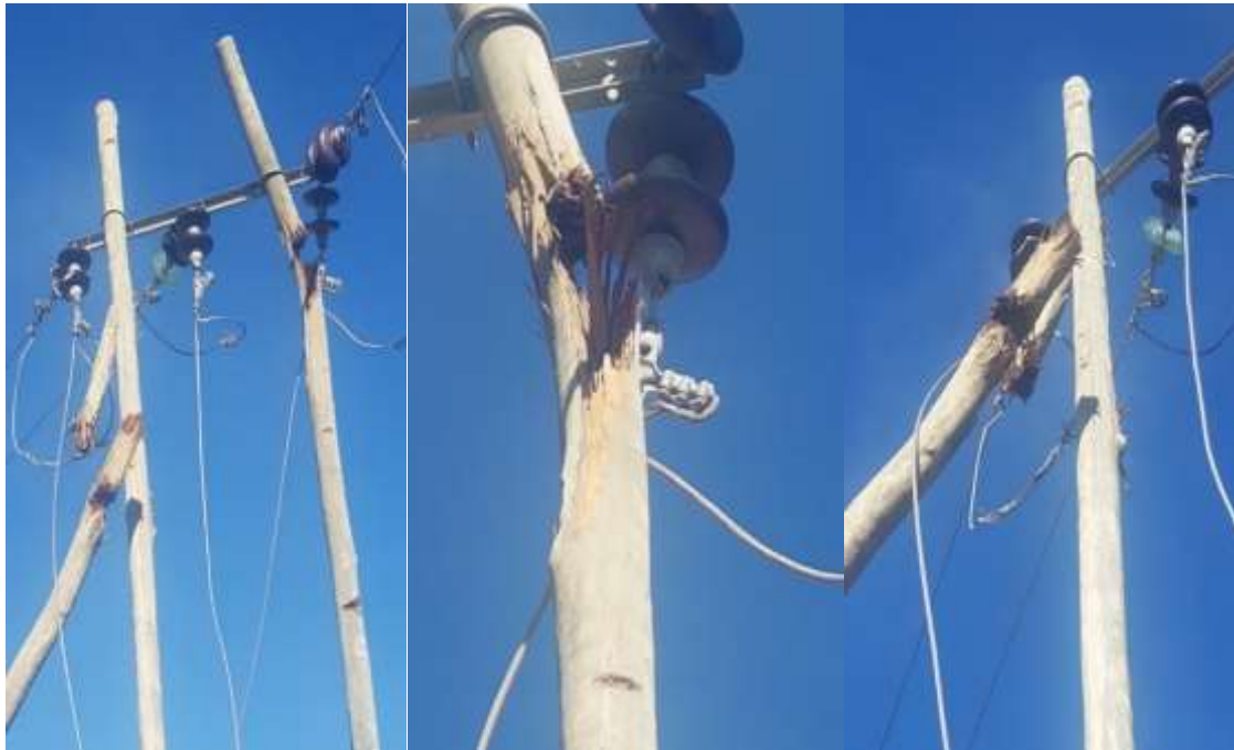
Fig.4.2: Feeder line support wooden poles and bush insulators failed due to the war in Tigray [38]
