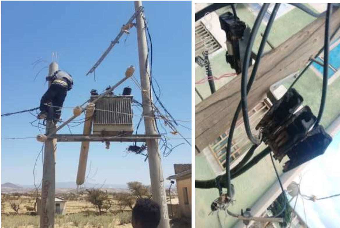
Fig.4.3: Feeder line transformer support and drop out fuse damage [38]
