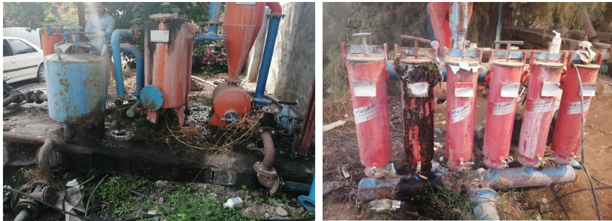
Fig. 5 Poor Condition of the Central Control System
