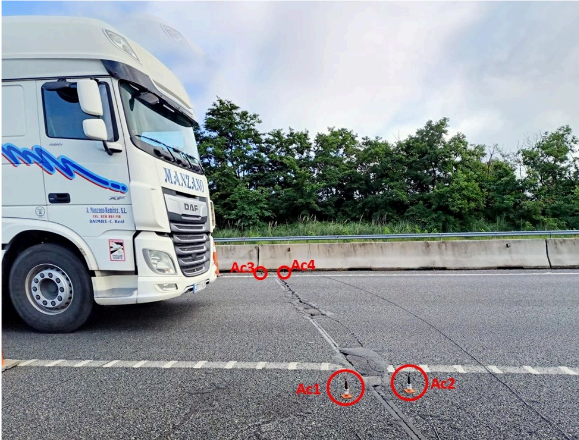
Figure 8. System of sensors arranged in the flexible road surface joint.
