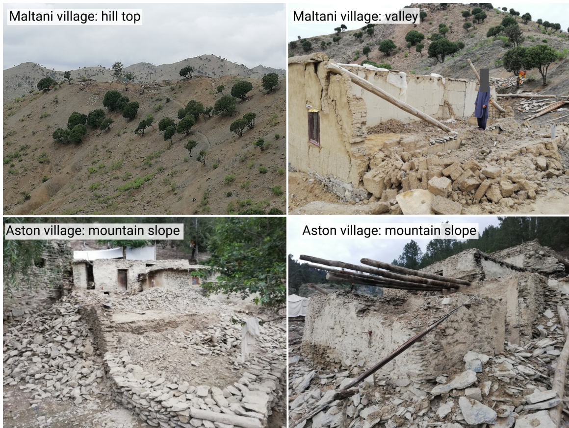
Figure S14: Destroyed houses near field site 1 and 2 (Maltani village; top) and field site 3 (Aston village; bottom). At Maltani village, many of the houses were built along the hillslopes or on the mountain tops; some houses were built in valleys. In this village, all houses were fully or partly destroyed, even though a few roofs were made with steel beams. At Aston village, houses, which were built at the hillslopes were mostly destroyed, while houses built in the valley suffered damage but were not completely destroyed. At the Maltani and Aston villages 17 respectively 2 people were killed.
