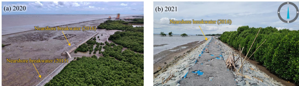
Figure S7. (a) Nearshore breakwaters constructed in 2015 and 2016 at Ban Khlong Hong Thong coastline (Sta.31+860–Sta.32+220) effectively trapped sediment behind the structures resulting in mangrove rehabilitation. On the other hand, these structures obstructed mangroves from colonizing further seaward. (b) Mangroves fully occupied the lee side of the nearshore breakwater constructed in 2016 within one year (2020–2021). The structure trapped approximately 1-m high sediment after five years from construction.
