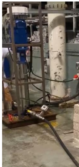
Pump, flow meter and hose pipe
