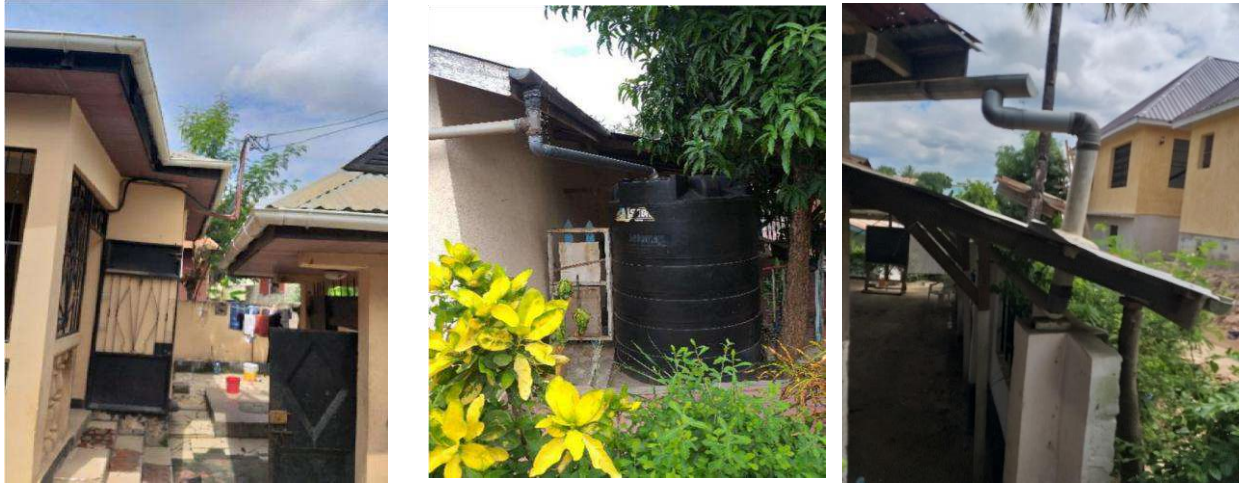
Figure 2 Rainwater Harvesting system at the visited site.
