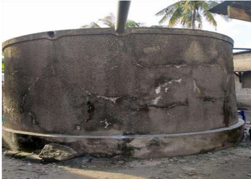
Figure 4 Cracks and leakages in storage tanks (Source: Researcher field visit)
