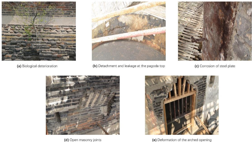
Fig. 3. Main deterioration types and representative pre-maintenance manifestations of the Yunyan Temple Pagoda:
