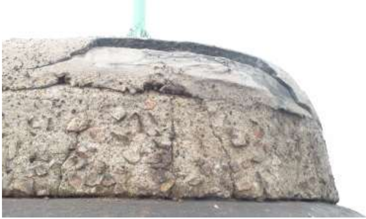
Cracking and detachment of the protective coating around the lightning-rod installation point
