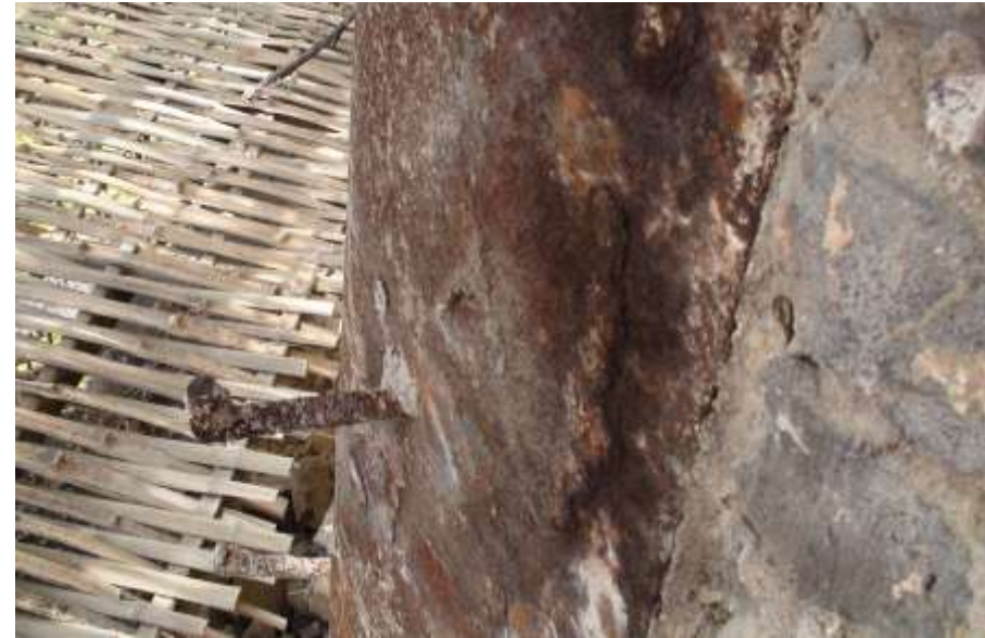
Mild surface corrosion before treatment
