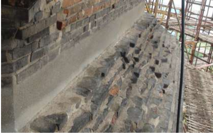
Before local repair
