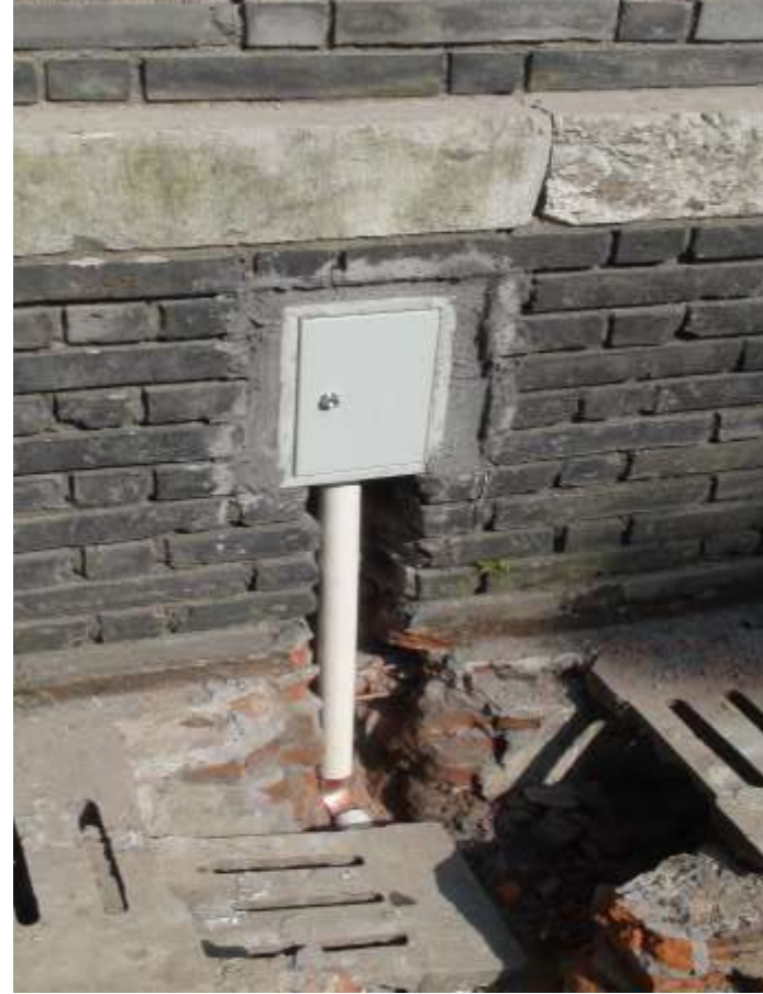
Lightning-protection inspection box
