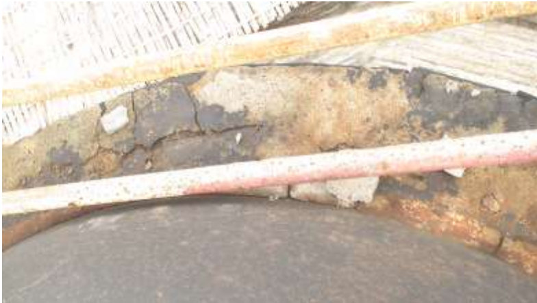
Detachment of the protective surface layer from the inverted-bowl element of the finial
