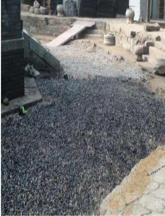
Insulated asphalt backfill for step-voltage protection
