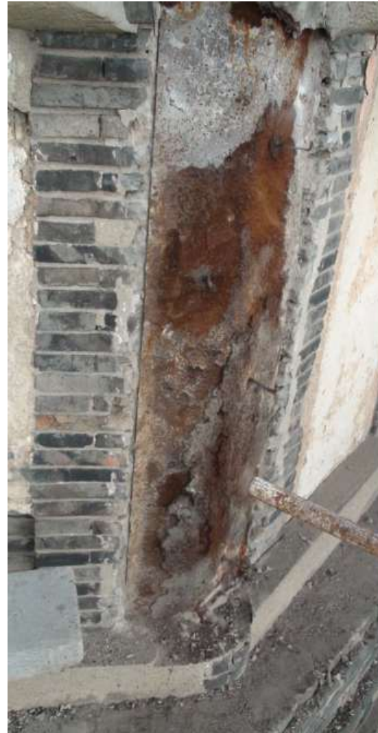
Severe corrosion of the steel plate within corner masonry column No. 5 at the fourth level
