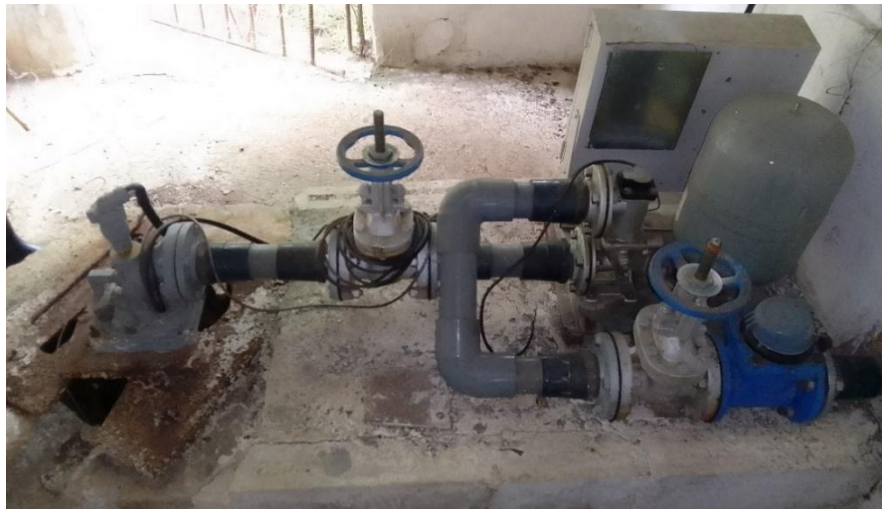
Fig. 2 Pumping system at the 14 July organoponic farm
