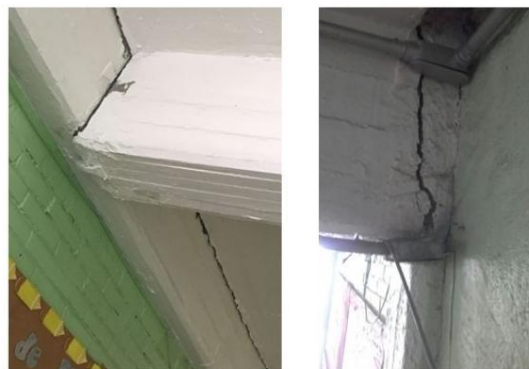
Figure 5. Damages at the School Tehuacán
