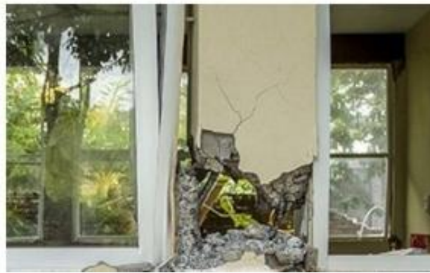
Figure 4. Damages at a column in School Tetela del Volcán
