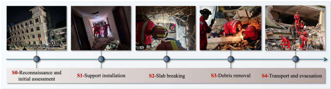
Fig. 8. Collapse condition and rescue operations at the Golden Country Hotel (photograph courtesy of Wen Bai).
