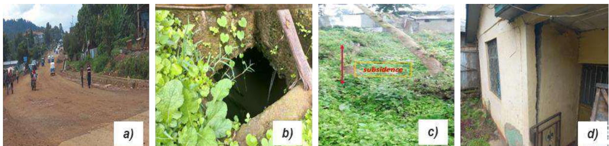
Fig.2 Photos showing instability section along Km2+520-2+660, Bonag-1
