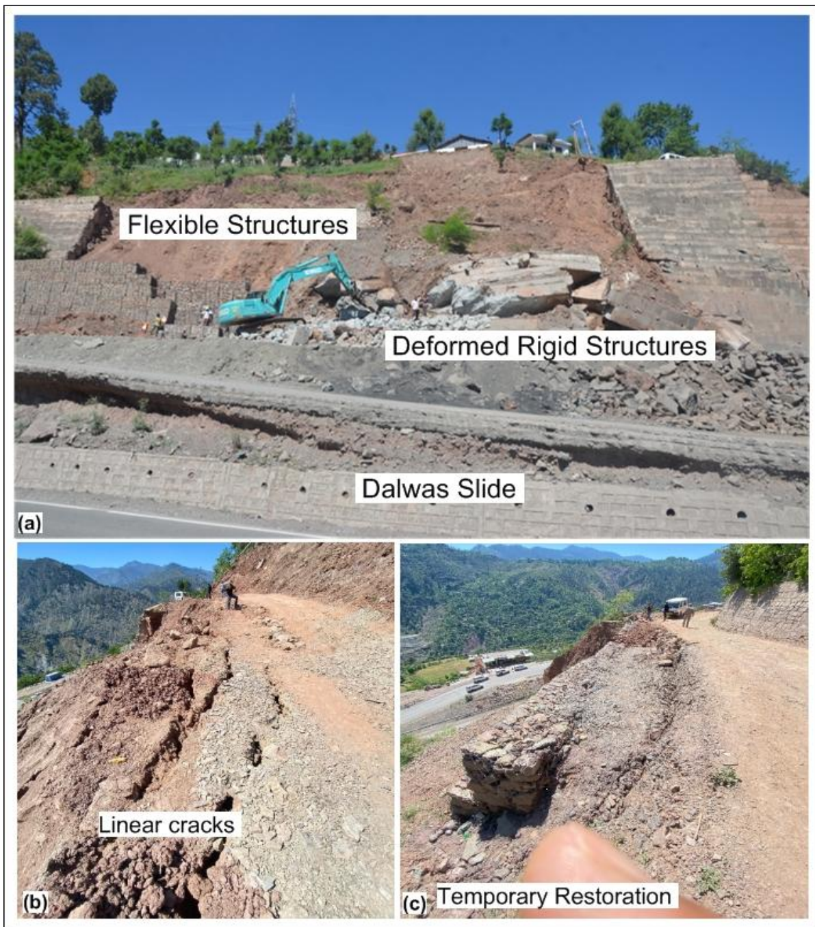
Fig. 6. Photographs showing (a) landslide along Jammu-Srinagar national highway at Dalwas, (b) linear cracks along the Dalwas-Karma Road, (c) temporary restoration works carried out on the Dalwas-Karma Road.
