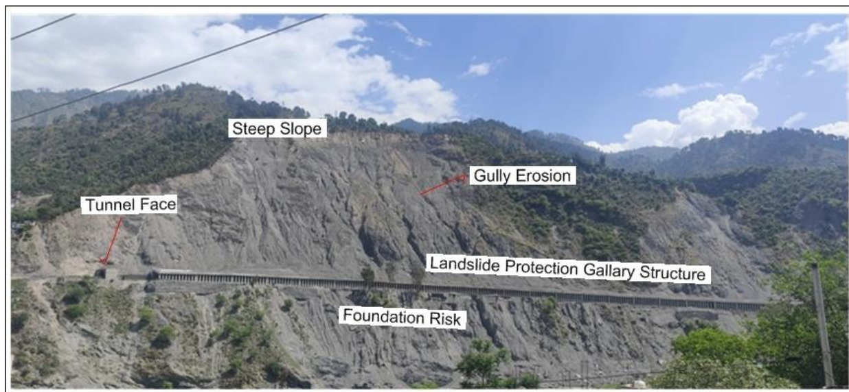
Fig.4. Photograph showing the Cafeteria Morh landslide and the associated engineering structure along a vital road connectivity corridor.
