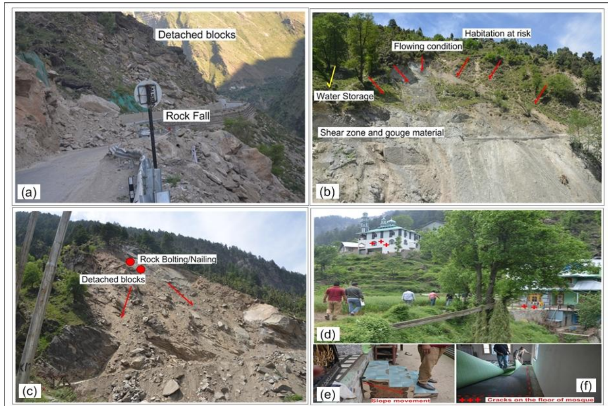
Fig. 7. Photograph showing (a) active landslide (rockfall) site at Drabshallah (b) landslide near Noos nallah, depicting downslope movement of material (c) rockfall at Pathar Nakki, where structurally controlled granitic gneiss slopes dip towards the road-cut, promoting planar failures and rock detachment (d) Dangdoru village along the Maru Sudhar River near the hydropower project site, (e-f) depicting localized minor structural subsidence, and deformation in the toe-strengthening wall.
