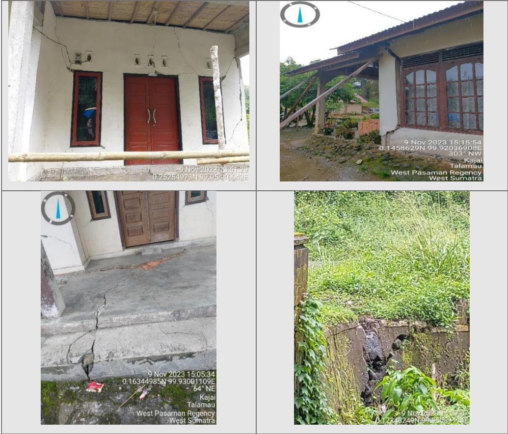
Fig. 9 On-site documentation of damage caused by the 2022 Pasaman earthquake
