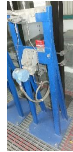
(b) Unit 4 Feedwater Flow Meter
