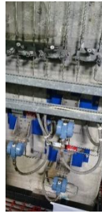
(a) Unit 3 Feedwater Flow Meter
